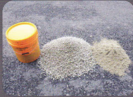
1. Prepare and weigh raw material (Cold Mix binder, quarry dust / sand & chip stones)
